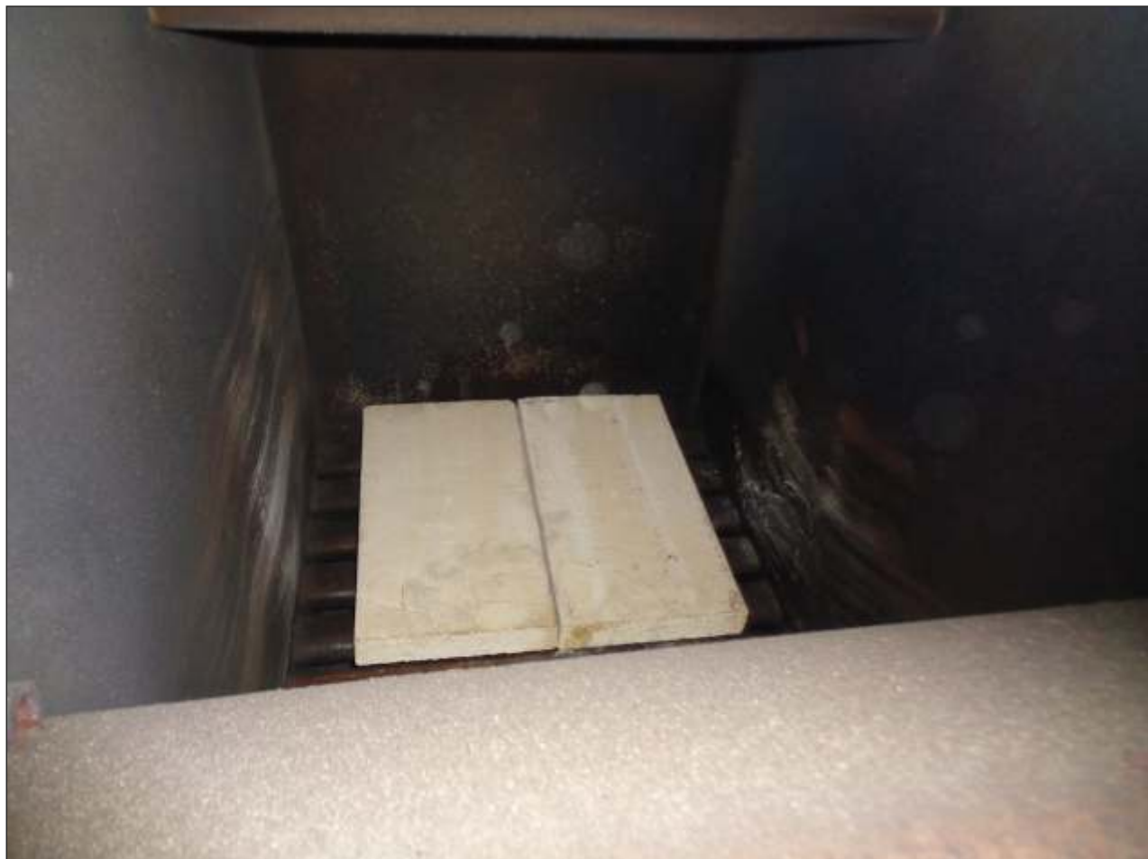
Picture 5: Position of fireclay plates on top of the grate in the firebox.
