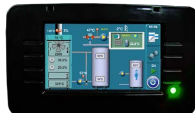
Multifunctional controller with a touch screen
