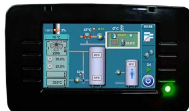
Multifunctional controller with a touch screen
