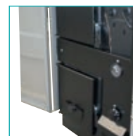
Kotlovska vrata, termomanometar, regulator propuha
